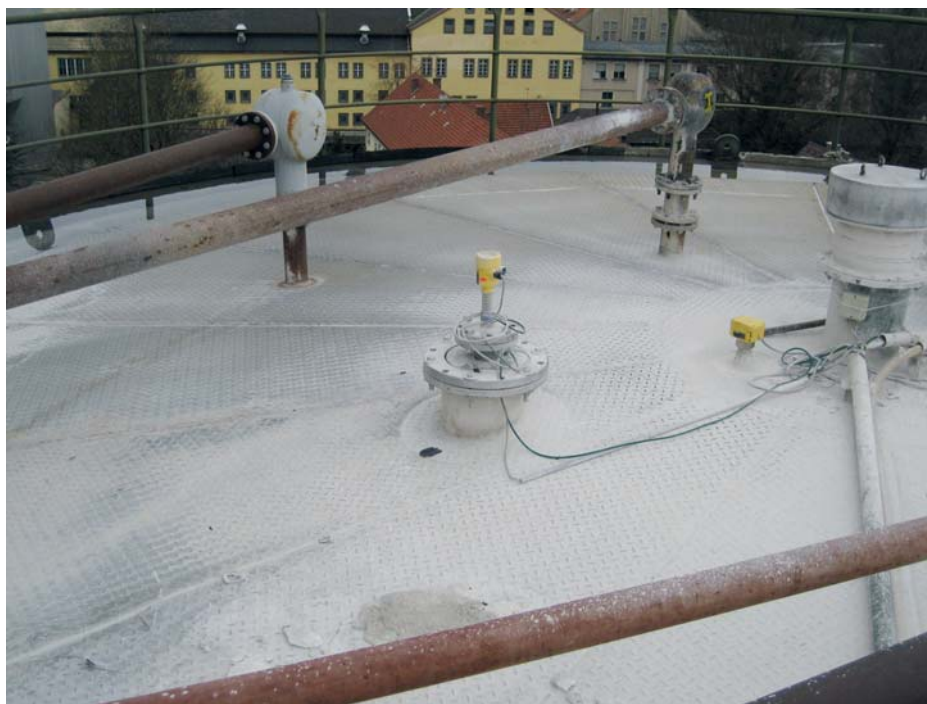
Fig. 5: Radar level measurement (picture middle) and capacitive max. detection (on the right) in the ash silo. Above and below in the picture the pneumatic filling pipes are recognizable
