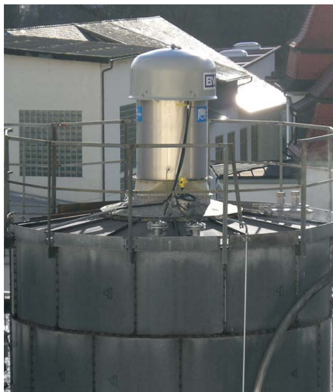
Fig. 4: Radar level measurement in the starch silo
