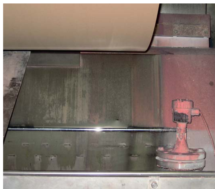
Fig. 2: Radar level measurement in the pulper below the tambours
